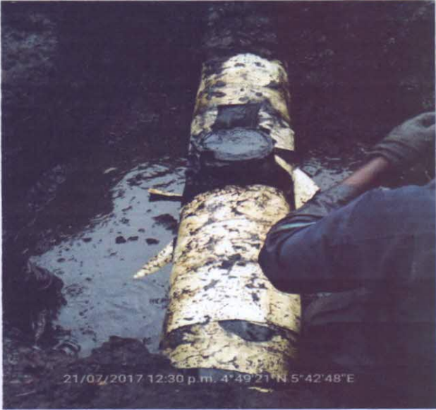
FIG 2: Spill point on excavation
